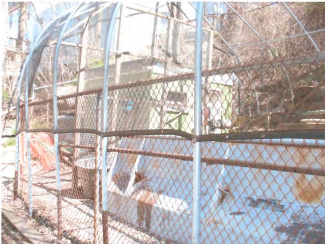
27 SEWER TREATMENT PLANT: NORTHEAST VIEW
