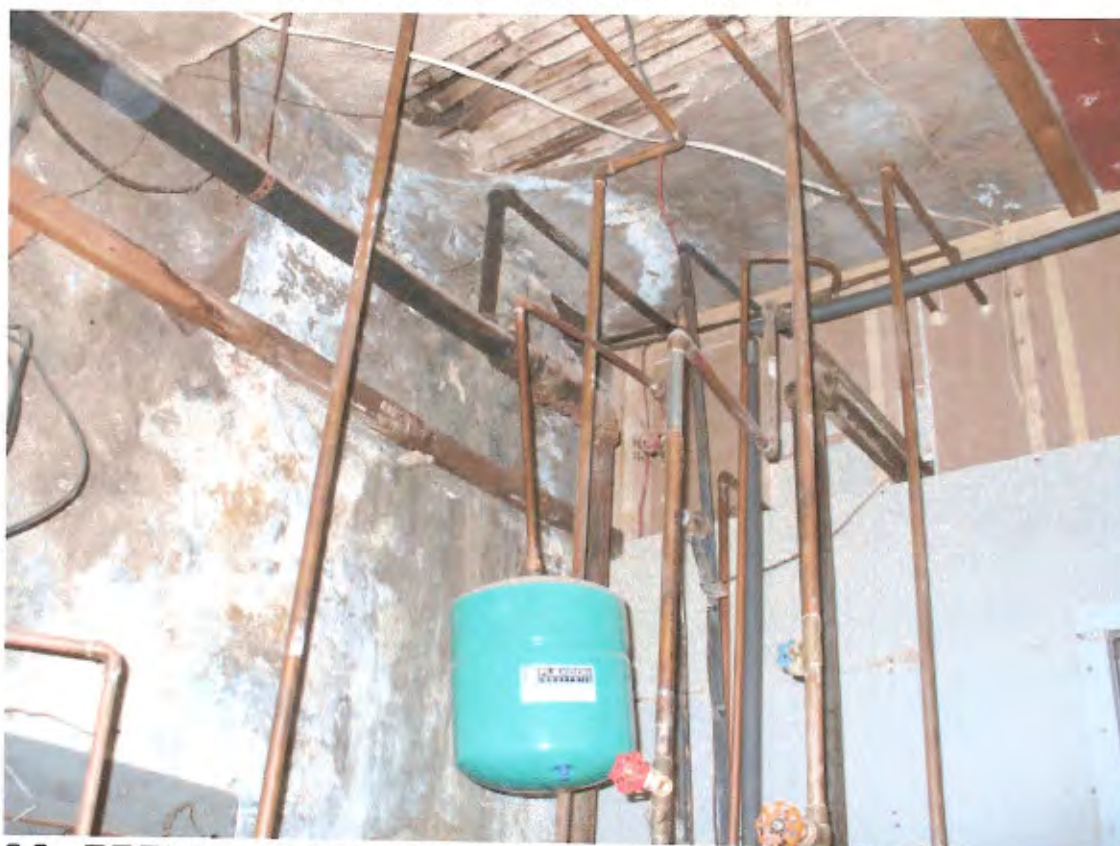
22 OFFICE: BASEMENT BOILER ROOM PIPING
