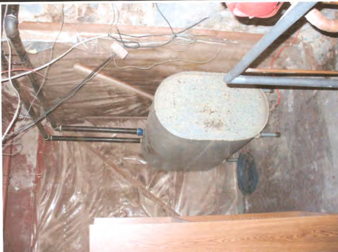
23 OFFICE: BASEMENT AST IN BOILER ROOM
