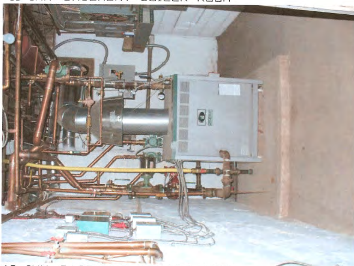
12 INN: BASEMENT UTILITY ROOM
