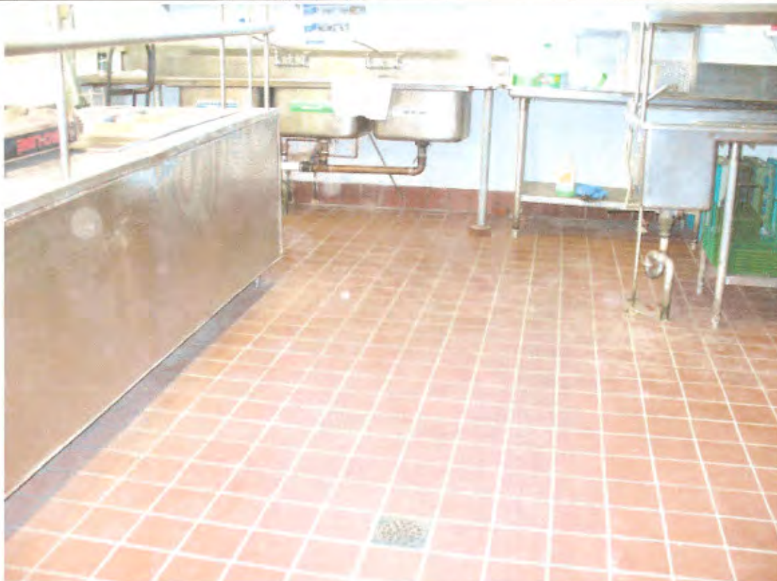
13 INN: MAIN FLOOR KITCHEN FLOOR DRAIN
