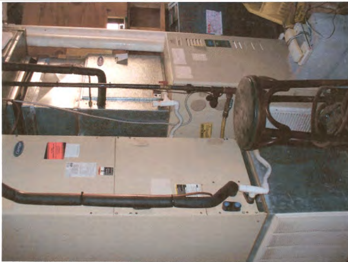
11 INN: BASEMENT BOILER ROOM
